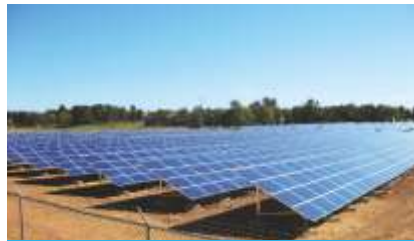
USA Lincoln County 6.97MW Solar Power Station
