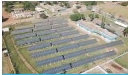
Brazil Imbauba 420kW Solar Power Station
