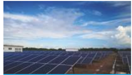
Brazil Santelisa 2MW Ground PV Plant
