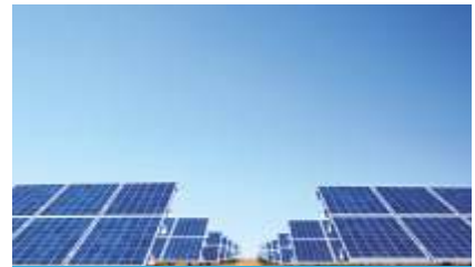
USA Kings Mountain 8MW Solar Power Station
