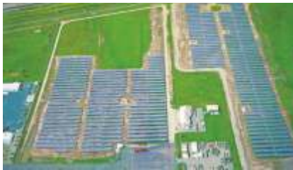
USA CA Depot Park 3MW Solar Power Station
