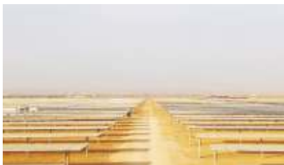
Jordan Mafraq 61MW Solar Power Station
