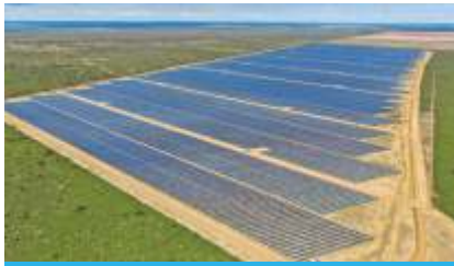
Brazil Barreiras 50MW PV Plant
